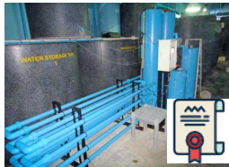
Tubular denitrification reactor For marine aquarium (2012)
