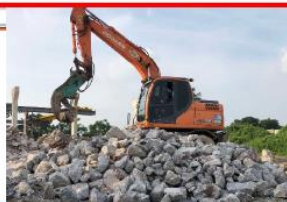
Stationary CDW crushing machine installed in Dong Anh District, Hanoi
